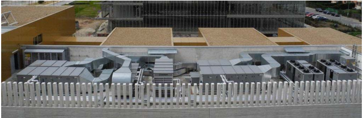
General view of the technical space on top of the laser bay
